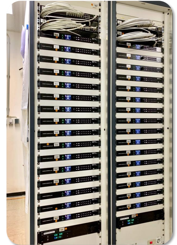
Fully redundant Multiplex Center with 258 DAB+ Encoders at NDR
